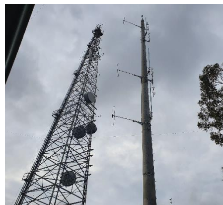
Monopole with 6/2/70/23 antennas.
